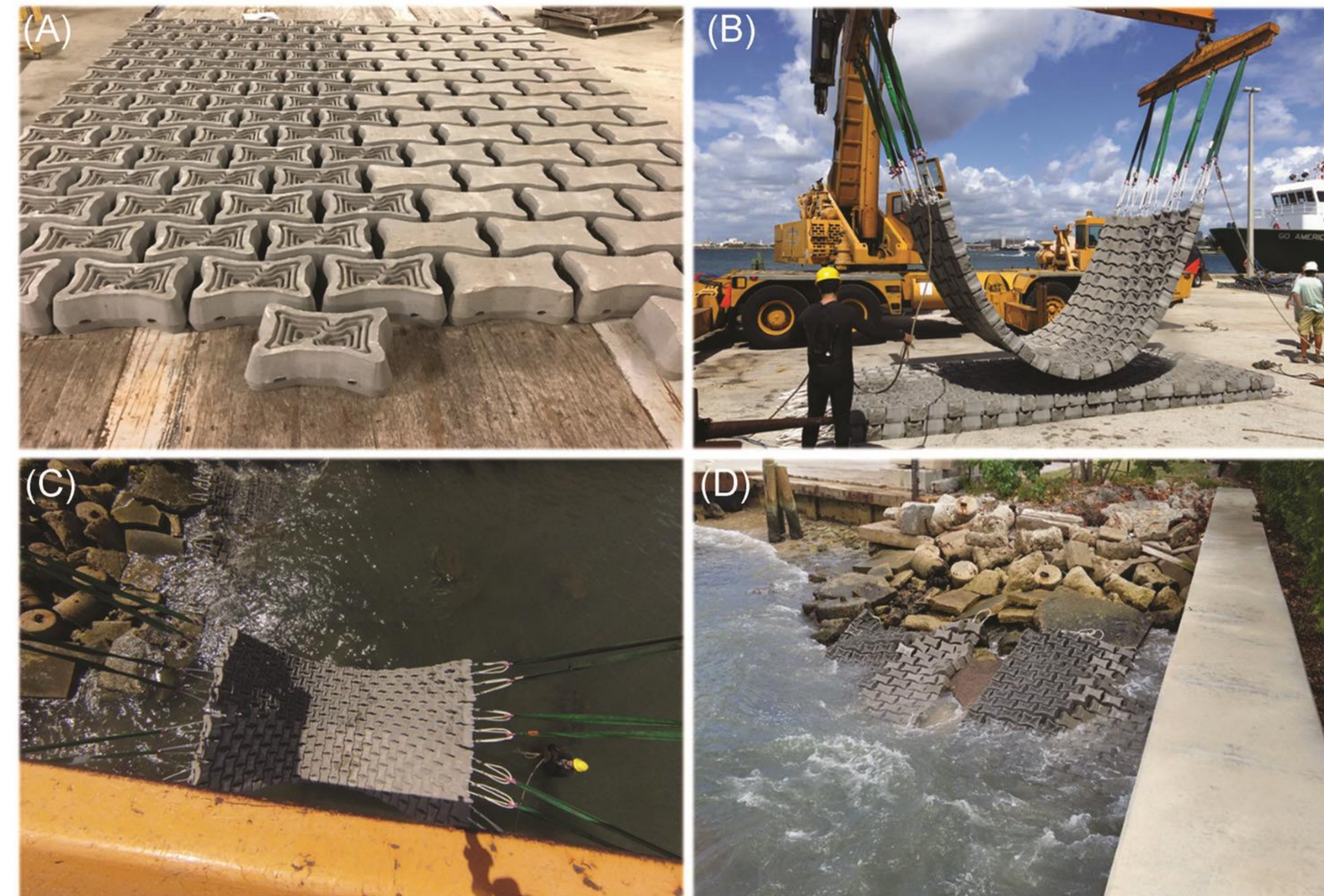
Manufacture and installation procedures of the Articulated Concrete Block Mattress. (A) Lacing the blocks to form half-textured ECO blocks (treatment) and half featureless CEM-I-based blocks (control); (B) crane lifting; (C) lowering to the water; and (D) in place on the riprap with the tops aligned with the MHHW line.
