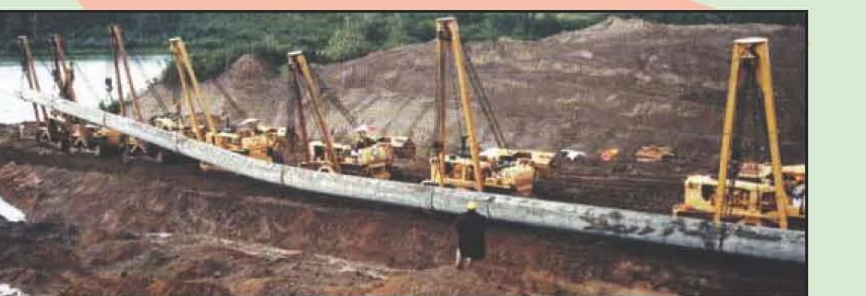
GH2 PIPELINE STORAGE
